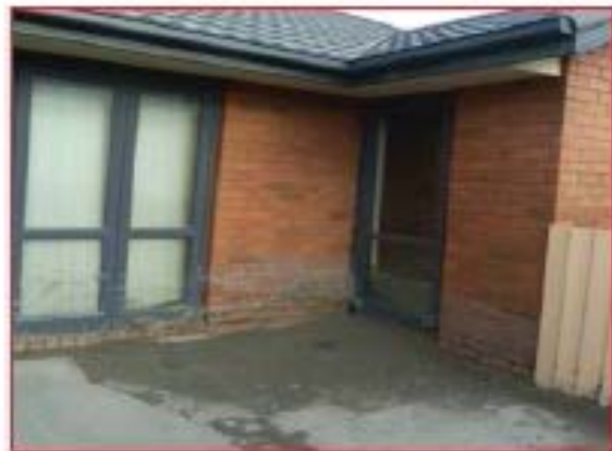
Outside of dwelling showing level liquefaction ejecta reached on brickwork and windows
