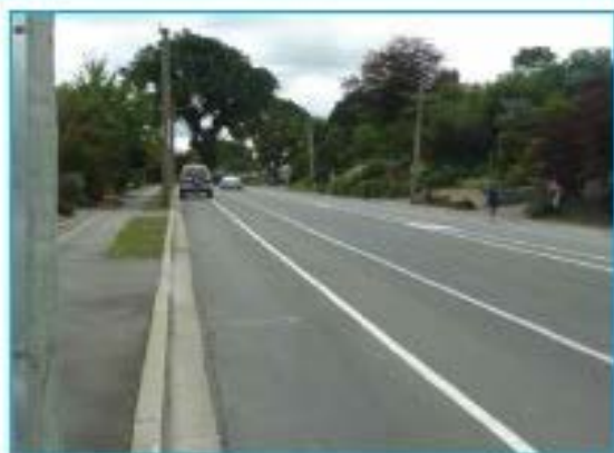
View of Centaurus Road with little damage
