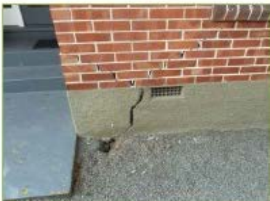
Foundation and brickwork damage
