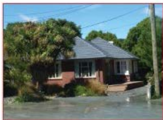
Foundation damage, tilting dwelling
